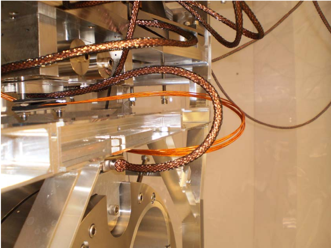
Figure 5: Routing and Clamping of Cables from UIM to PUM
