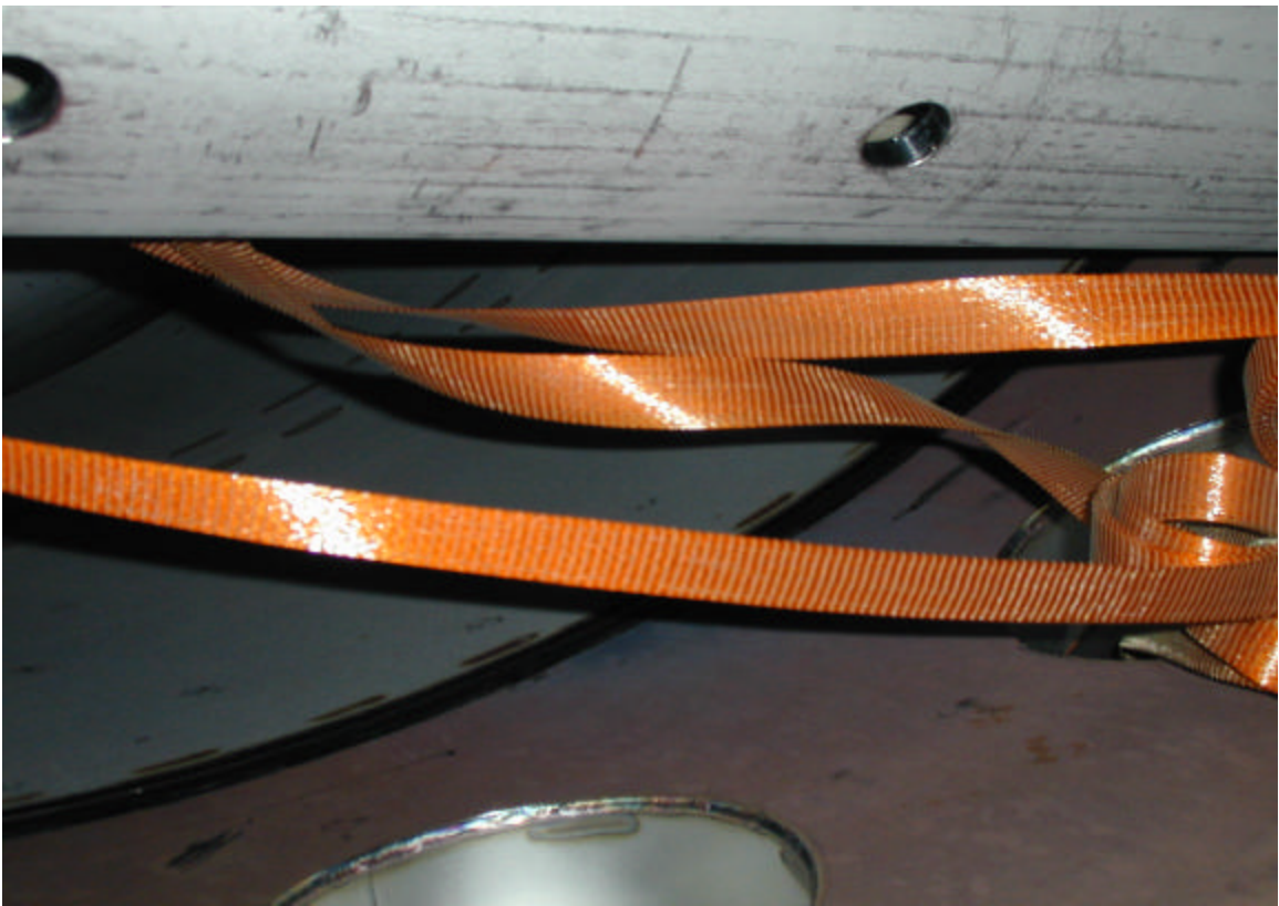
Looking up at cabling in seismic stacks.
