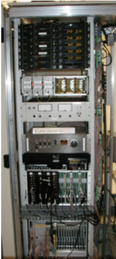
Figure 10: Photograph of 40-meter PSL electronics rack
