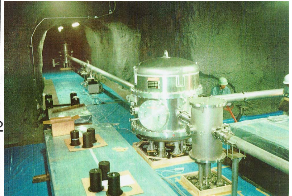
20m Prototype detector installed
