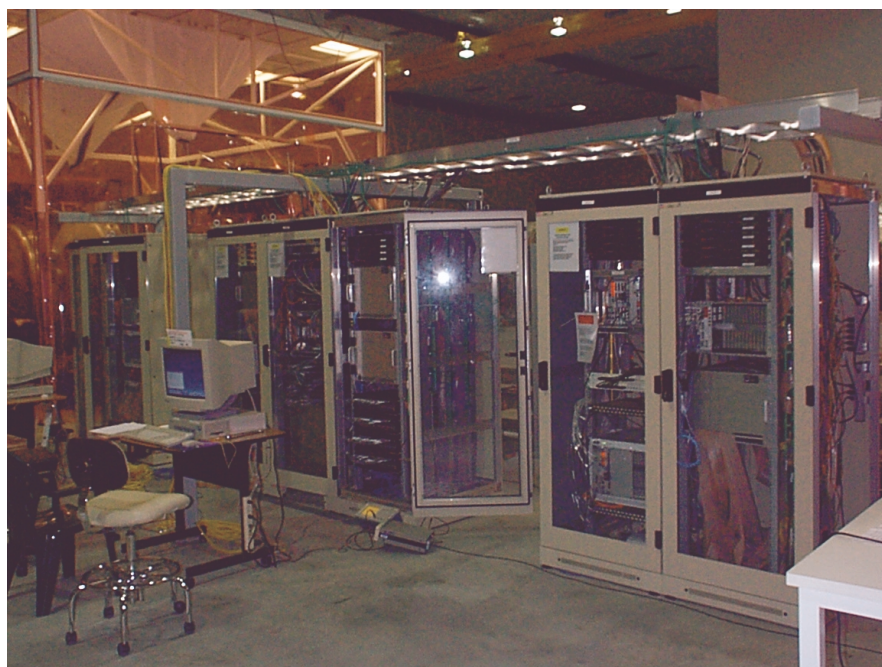
Control System Racks (2km Interferometer)
