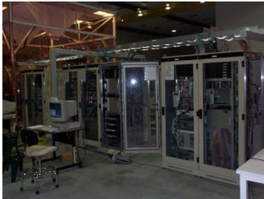
Control System Racks
