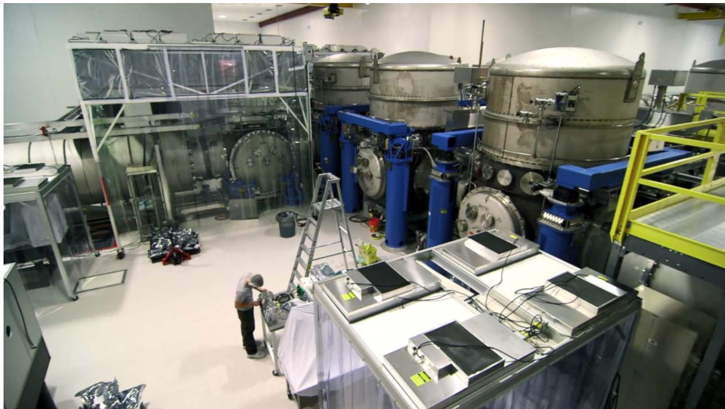
View inside the LHO Corner Station
