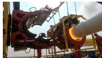
RF induction heating: Magnetic properties of mild steel make it more appealing for RF heating.
